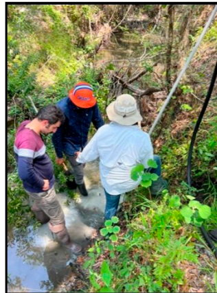
Members of Dr. Golmohammadi's lab installing a groundwater well for monitoring water quality.
