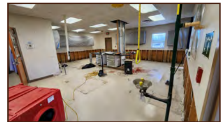
Forage and Soil & Water Lab bldg. after the flood damaged walls and cabinets were removed.
