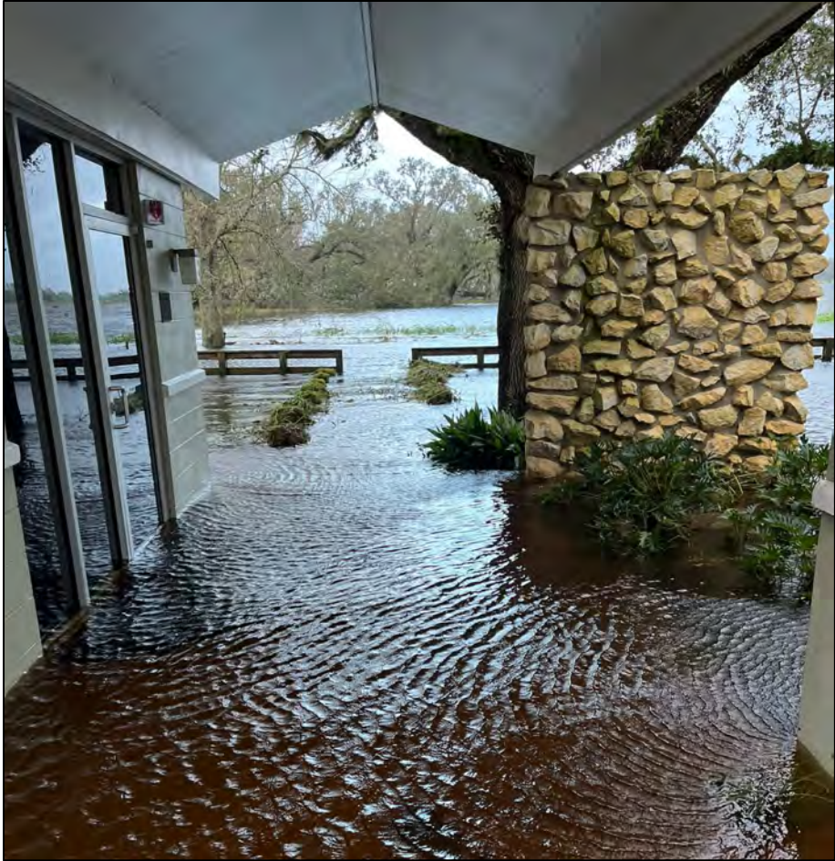
Flooding by the main office building the day after Hurricane Ian.
